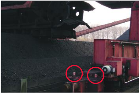
Lubrication of flange bearing on support rollers
