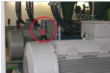
Lubrication of electric motor
