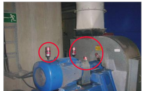
Lubrication of electric motor and shaft on a secondary air fan.
