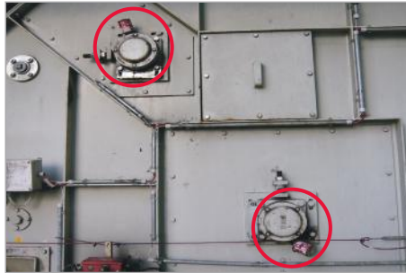
Lubrication of flange bearing on a bucket conveyor
