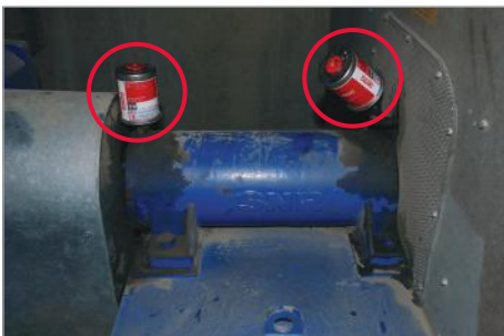
Lubrication of pillow block on fan
