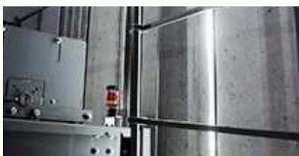
Lubrication of guide rails on counterweights
