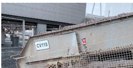
Lubrication of the bearing block on a drive disc
