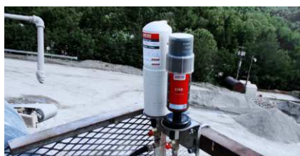
Lubrication of pillow block bearing on conveyor
