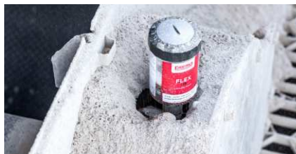
Lubrication of pillow block bearing on grit and sand screen
