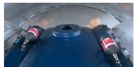
Blade bearing lubrication
